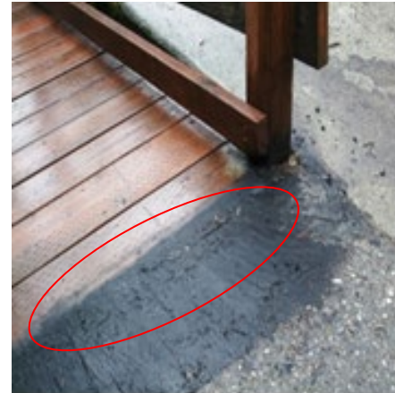
Asphalt Cold Patch is Used to Reduce This Threshold Edge (red circle)
