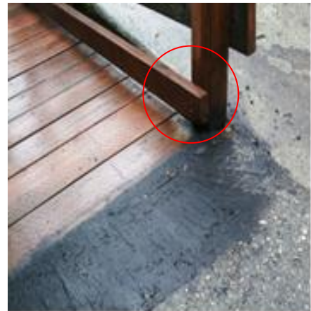
Ramp Edge Guard (red circle)
